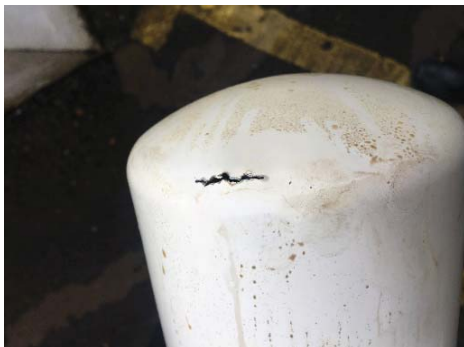
Figure 11. Leak on filter
